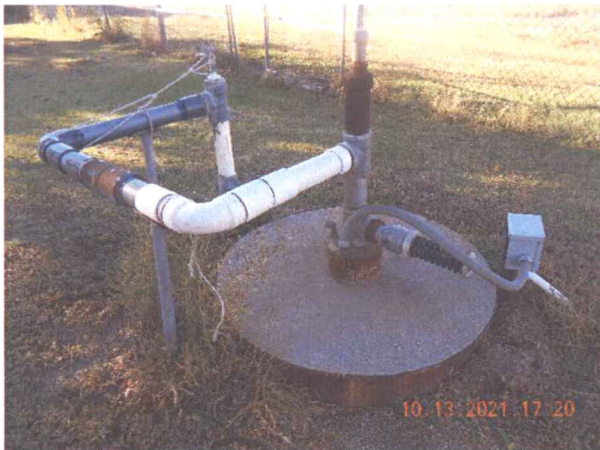
Well, east of storage tank 37.99578, -101.12139
