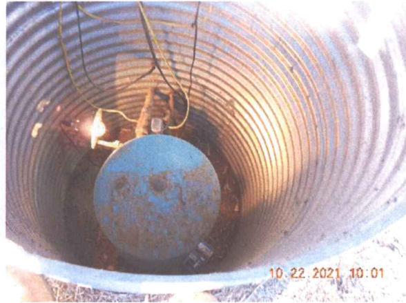
Inside well with hose
