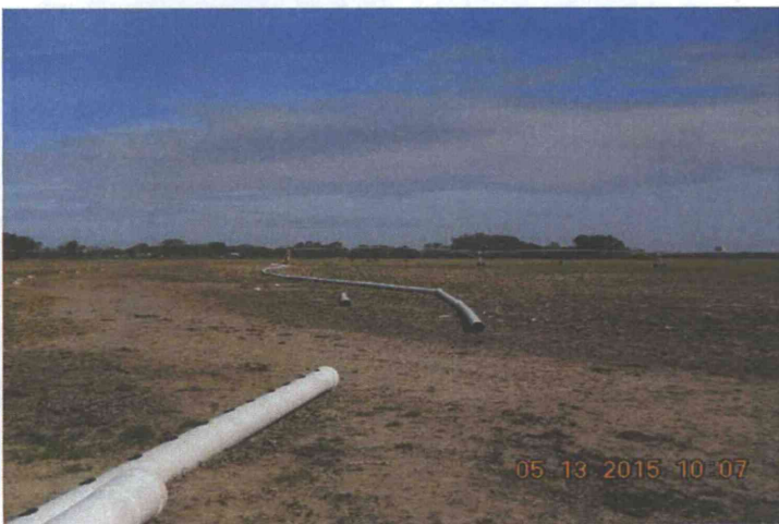
Pipe leading to center pivot in Northwest Quarter
