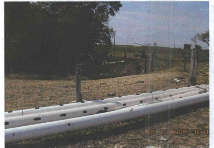
Pipe leading South possibly to South center pivot
