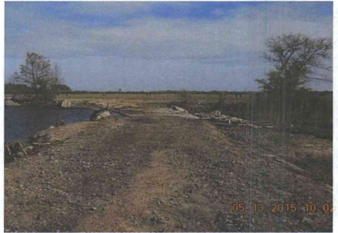
Right bank looking North at Obstruction
